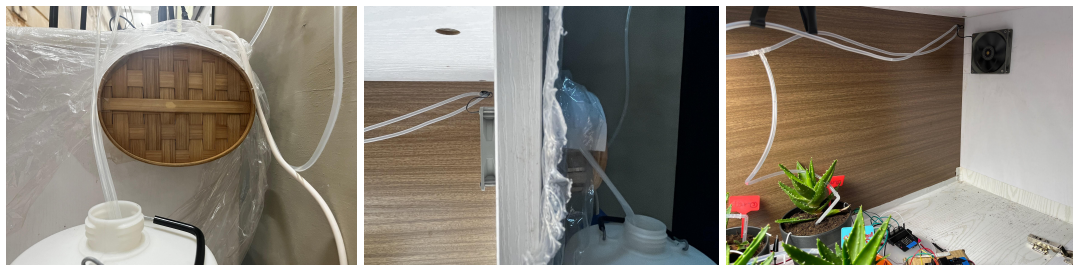
Fig. 2.33 Controlling the air velocity and ensuring ventilation: fan
